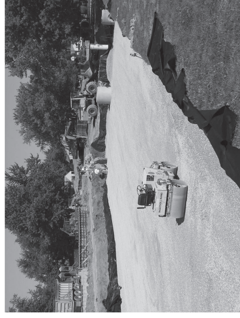
Place clean, crushed, angular stone foundation 6" (150 mm) min. Compact to achieve a flat surface.
