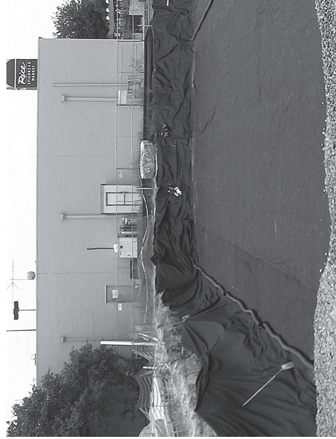
Place non-woven geotextile over prepared soils and up excavation walls. Install underdrains if required.
