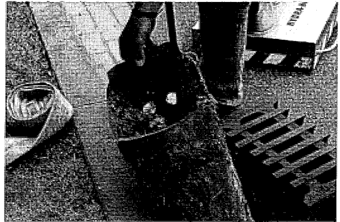
Debris from storm drains and catch basins should be collected and disposed of according to best practices and local regulations.
